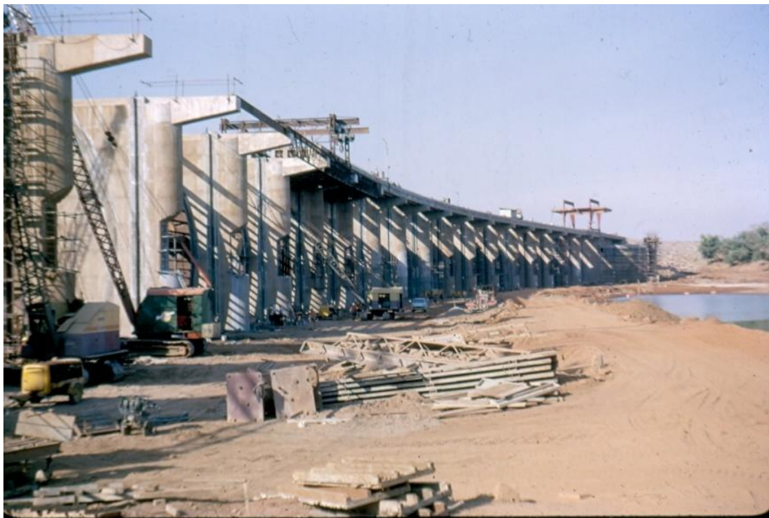
The Dam nears completion... all piers to full height... the roadway approaches the western abutment.
